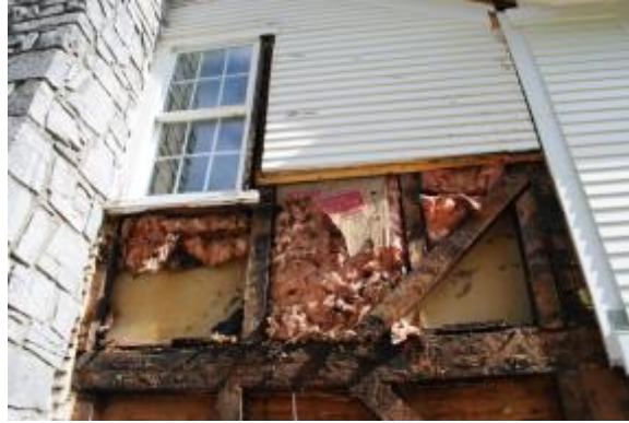
The house itself required extensive repair.
